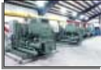
Centrifugal air compressors
