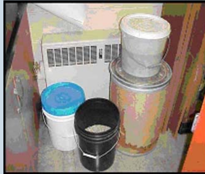
Chemicals stored next to the heater
