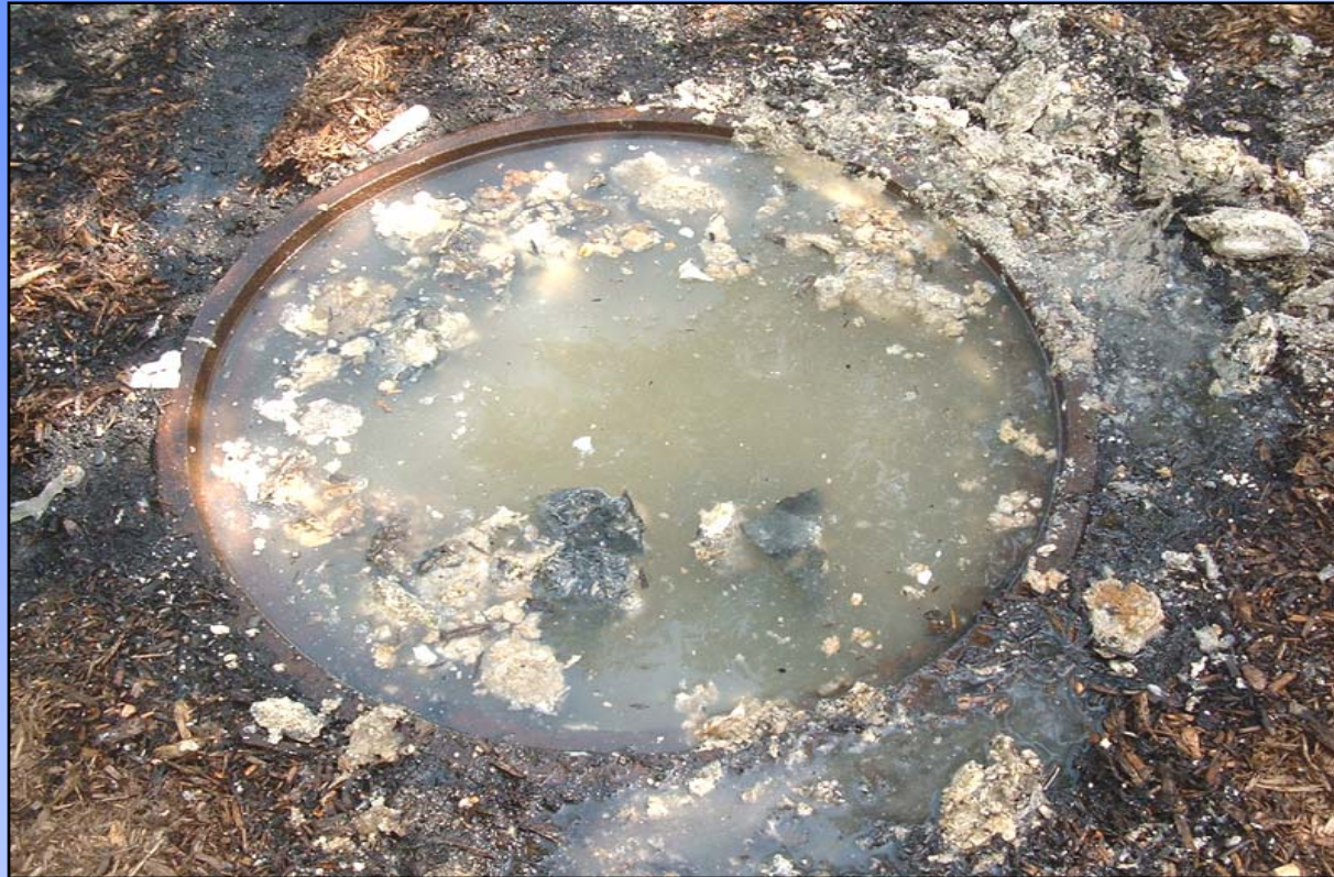
Blockage due to poor maintenance on Passive In-Ground Grease Traps
