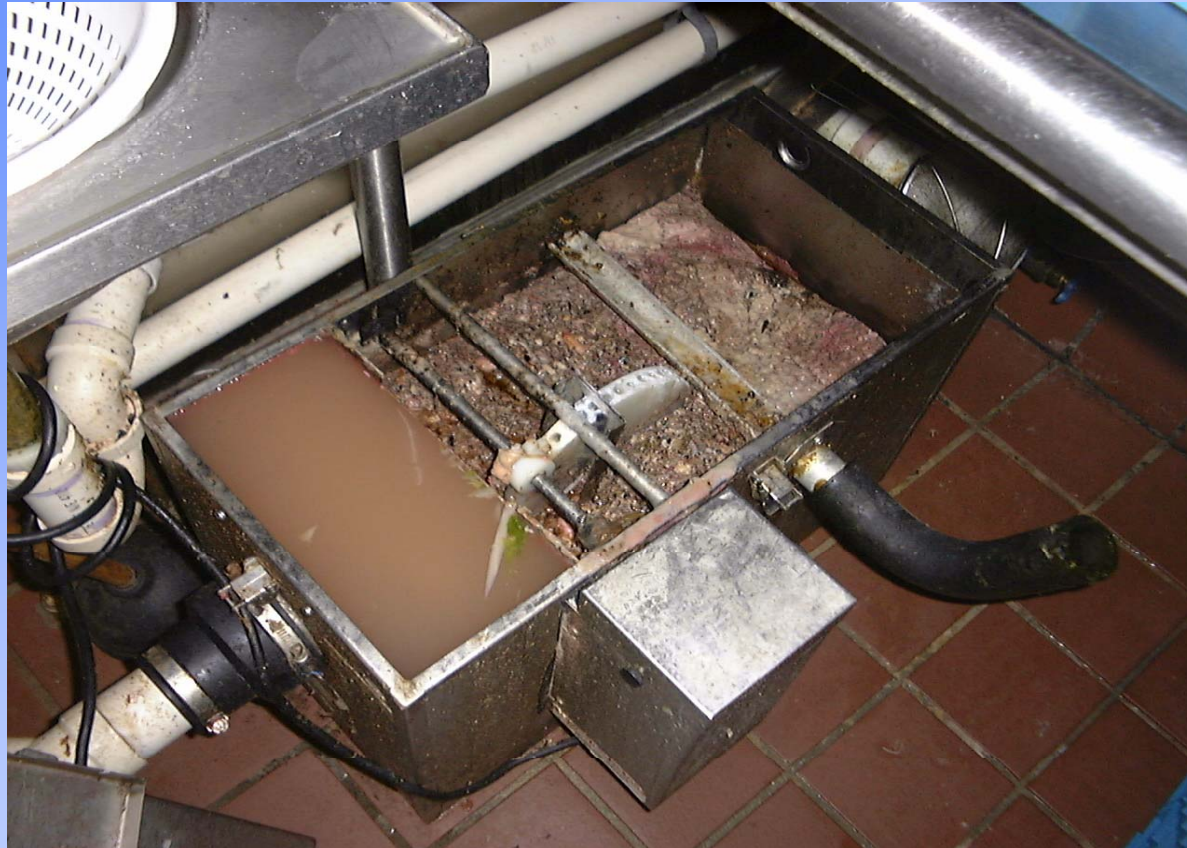
Poorly Operating Automatic GRU
